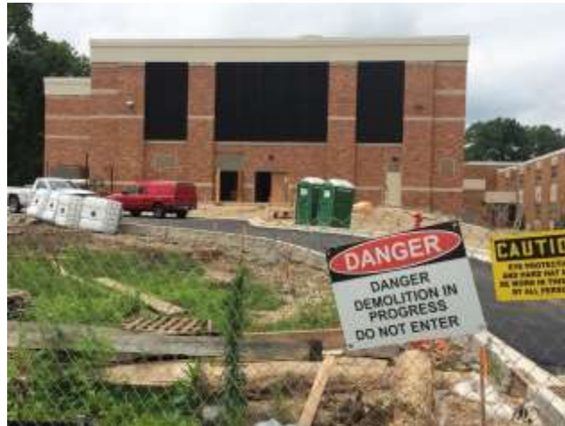
Construction of a new indoor swimming pool at Libertyville High School is nearing completion.
